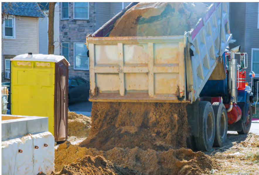
The best excess soil management outcome is when none is required. Creative and beneficial on-site reuse of excess soil should be top of mind.
